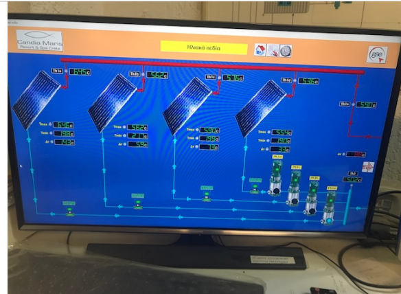
Solar panels measurements
